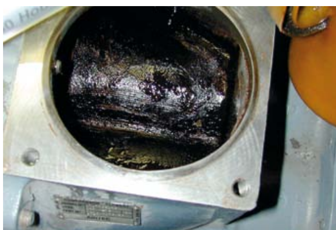
Residues in the compressor caused by oil
